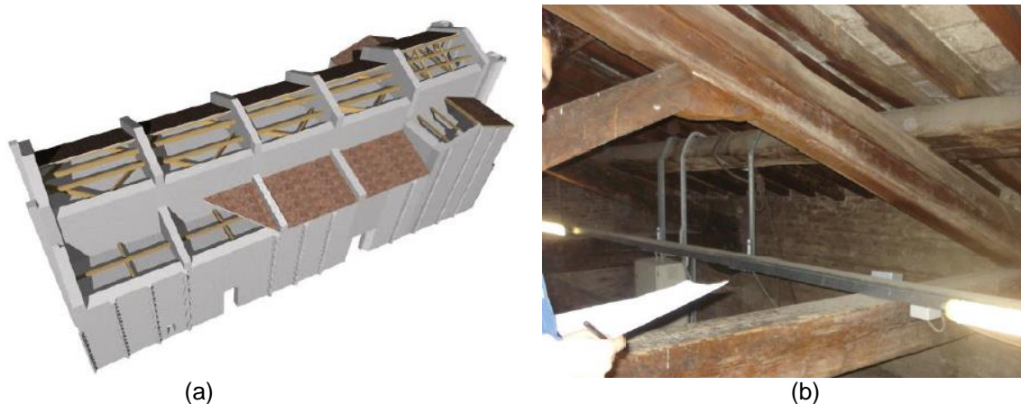
Figure 21: Structural elements in the case study Modena Cathedral. Roof and walls schematic representation (a); detail of roof structural elements (b).
