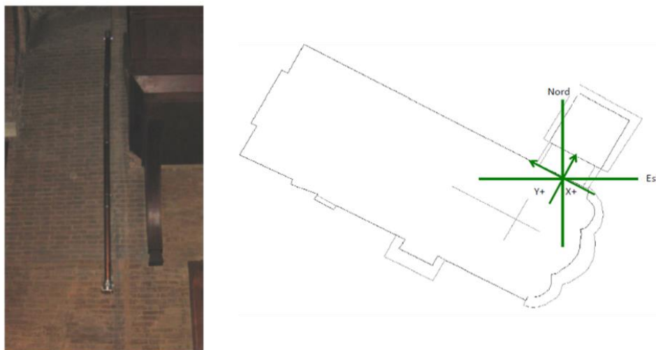
Figure 2.2.42: Inclinometer installed on the longitudinal wall of the cathedral (close to the buttress) FP1 and the conventional signs used.
