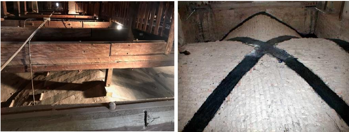
Figure 1.4.12: Application of FRP strips on the vaults of San Petronio church in Bologna and town hall of Assisi.
